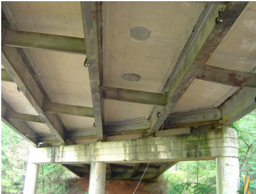
Lower photograph shows the instrumentation attached to the steel framing of a skewed highway bridge to provide data needed for the assessment and rating of the bridge.
