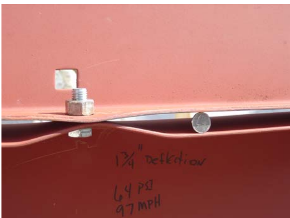
Photograph shows the impact damage to the wall system of a tornado shelter from a 15-lb 2x4 missile traveling approximately 100 mph.
