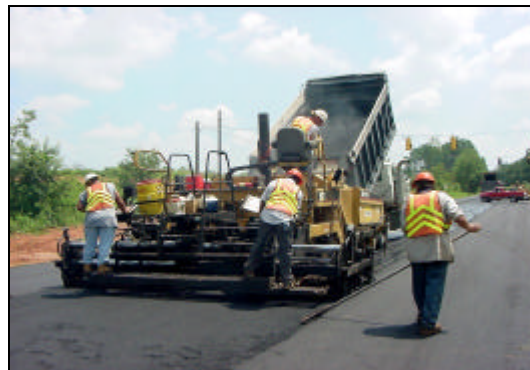
Asphalt pours from the dump truck into the paver and is laid at temperatures exceeding 300°F
