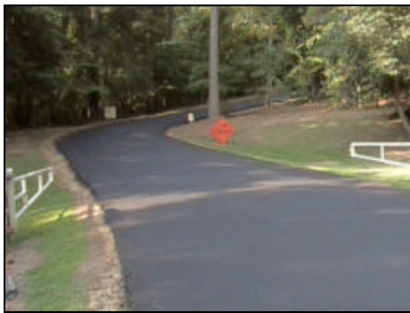
The Outdoor Laboratory access road on Clemson's campus is the first stress absorbing membrane interlayer (SAMI) constructed by ARTS.
