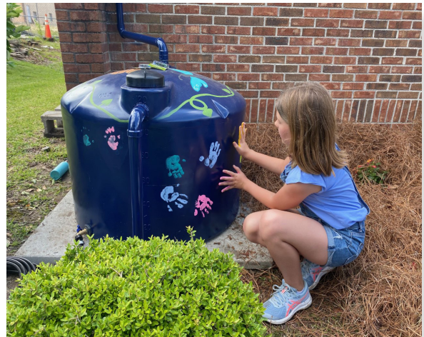
Community members help paint a 150-gallon cistern installed to capture rainwater from the roof of Andrews Public Library.
