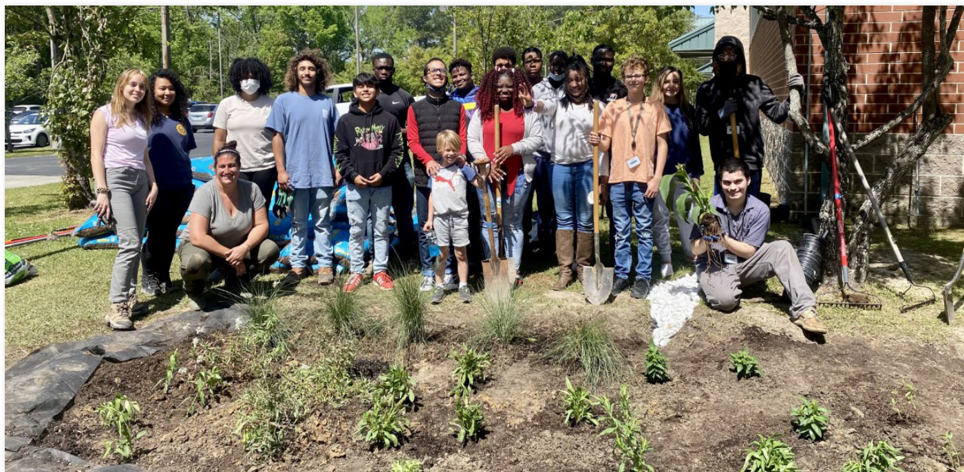
Students from Andrews High School helped install a rain garden at their school in partnership with The Nature Conservancy & Clemson Extension.
