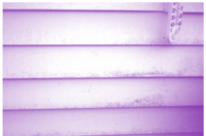
Figure 1. Mildew on side of house.
