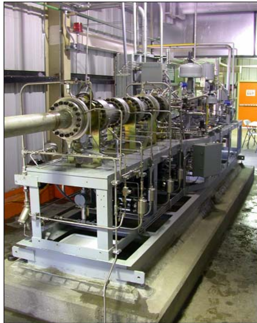
Figure 3. CES Demonstration GG, 170 MW t
