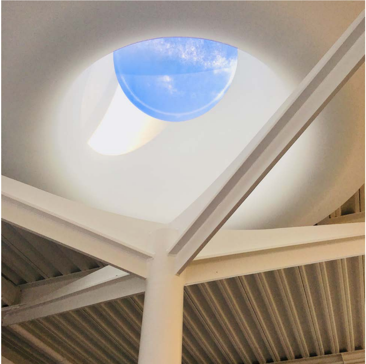
Lee 3 skylight. Thomas Phifer & Partners with McMillian Pazdan Smith Architecture. Photo D. Harding. Groundbreaking, April 23, 2010. Occupancy, Jan. 3, 2012.
