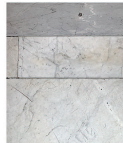
Example of White Marble Pavers in Genova
