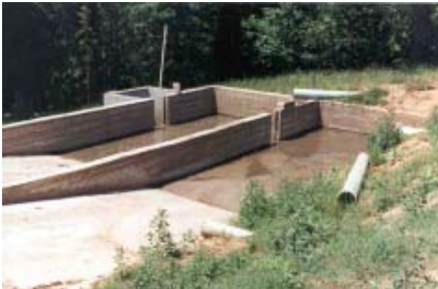
Figure 2. Two-chambered settling basin.
