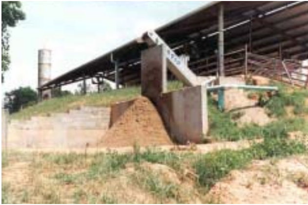
Figure 1. Inclined stationary screen and solids storage area.
