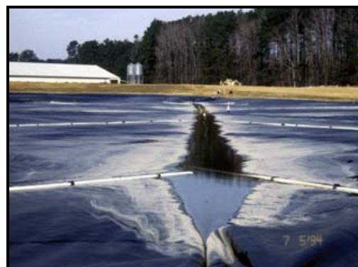
Figure 7. A covered lagoon digester (PSU, 2007).
