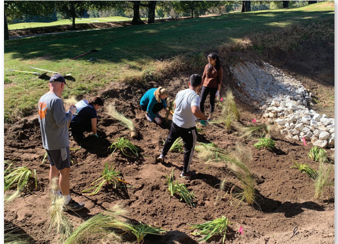
CU students & staff installing plants in a bioretention cell as part of Solid Green Day at Clemson University.
