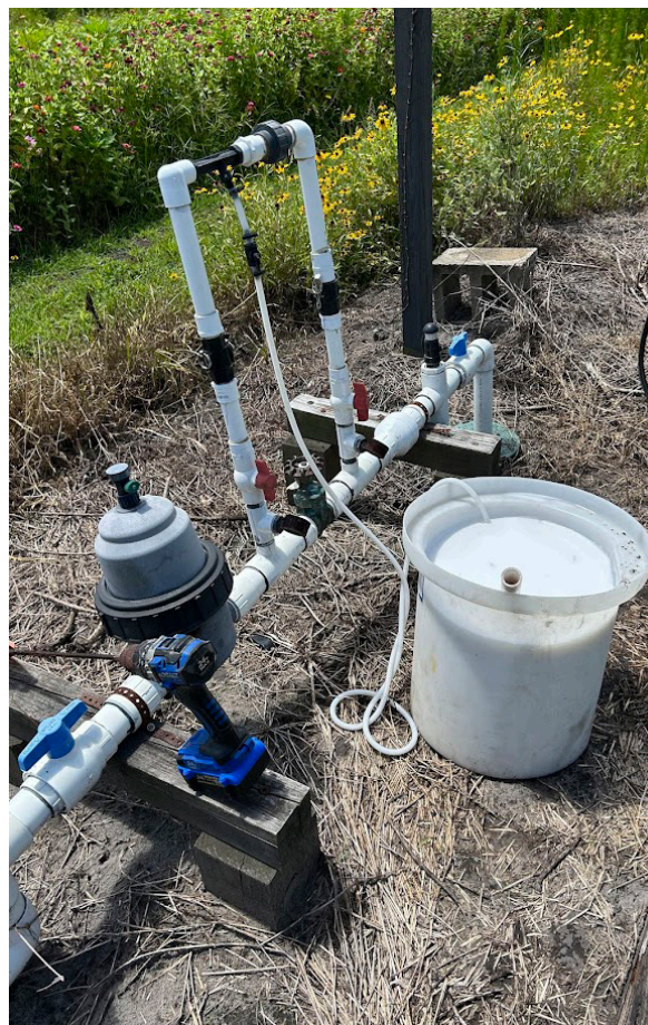
A venturi fertigation injector is a relatively inexpensive system that can deliver precise amounts of fertilizer to plants at just the right time
