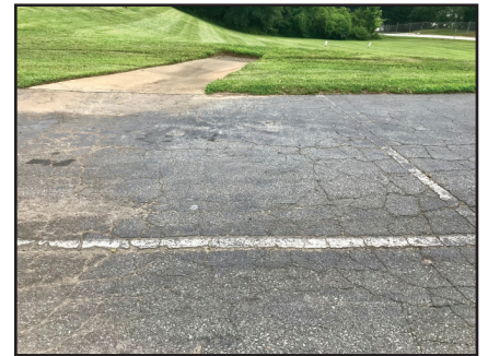
Parking lots that are directly connected to a storm drain, like this one here, can lead to heated runoff entering waterways.
