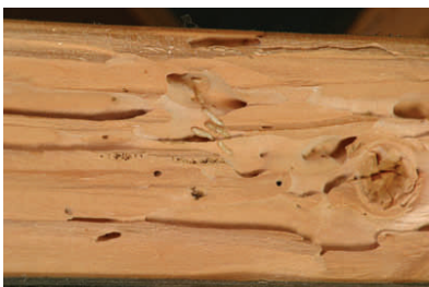
Drywood termite damage
