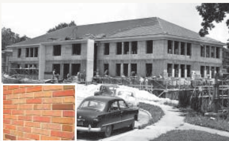
Construction of Olin Hall (About 1952) With a Light Range of Bricks (insert) Departing from the Red Brick Prevalence on Central Campus
