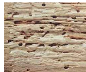
Powder-post beetle damage
