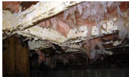
Wood-decaying fungi. damage
