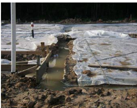
Chemical pooled in a footer of a water-saturated site.
