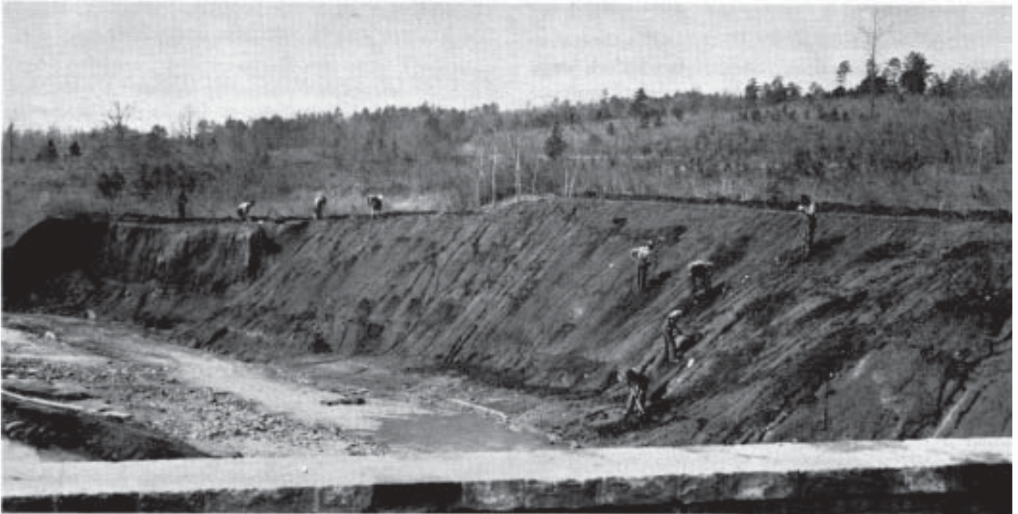
1940 photo of WPA (Work Projects Administration) workers preparing pot holes for kudzu plants on the banks of a stream. Soil from the banks was silting constantly into the water.
