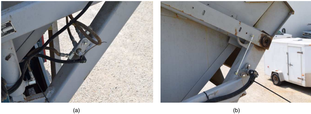
Figure 1. Pressure transducer (a) and rotary potentiometer (b) as installed on 2108 peanut combine.
